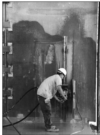
AN INSTRUMENT OF A DIFFERENT SORT: Part of the symphony of sounds emanating from the HPAC construction
