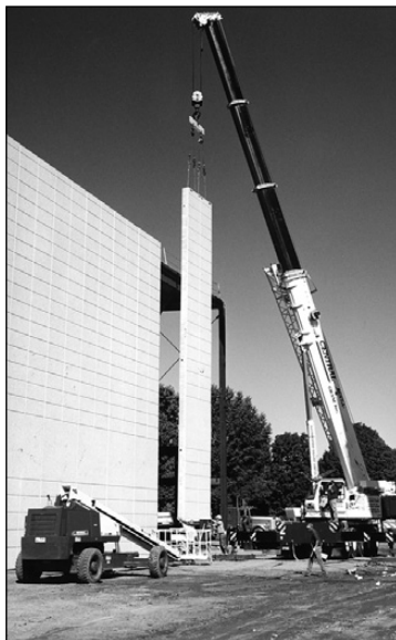
IF YOU BUILD IT. . . : A Fiskars' crane positions part of the outer wall of the HPAC.
